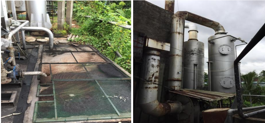
Figure 4: Water Treatment Plant
